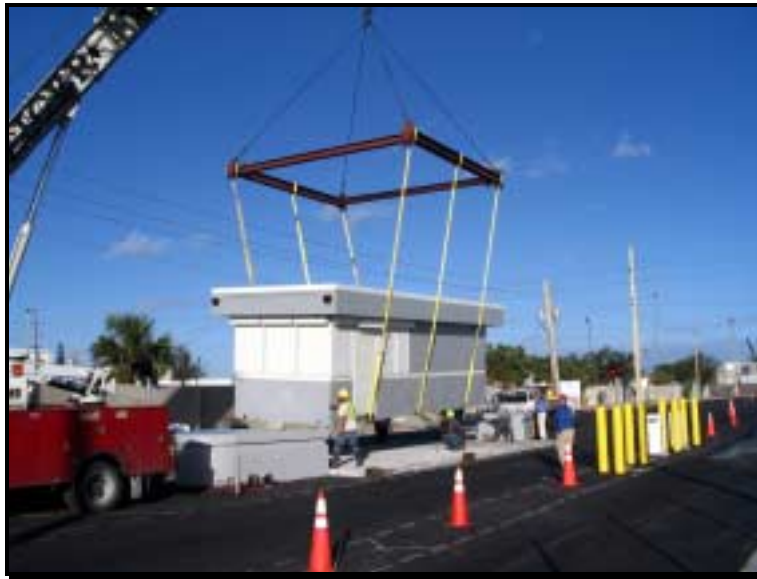
A new main gate is lowered into place at the Port's cargo entrance along Old Dixie.
